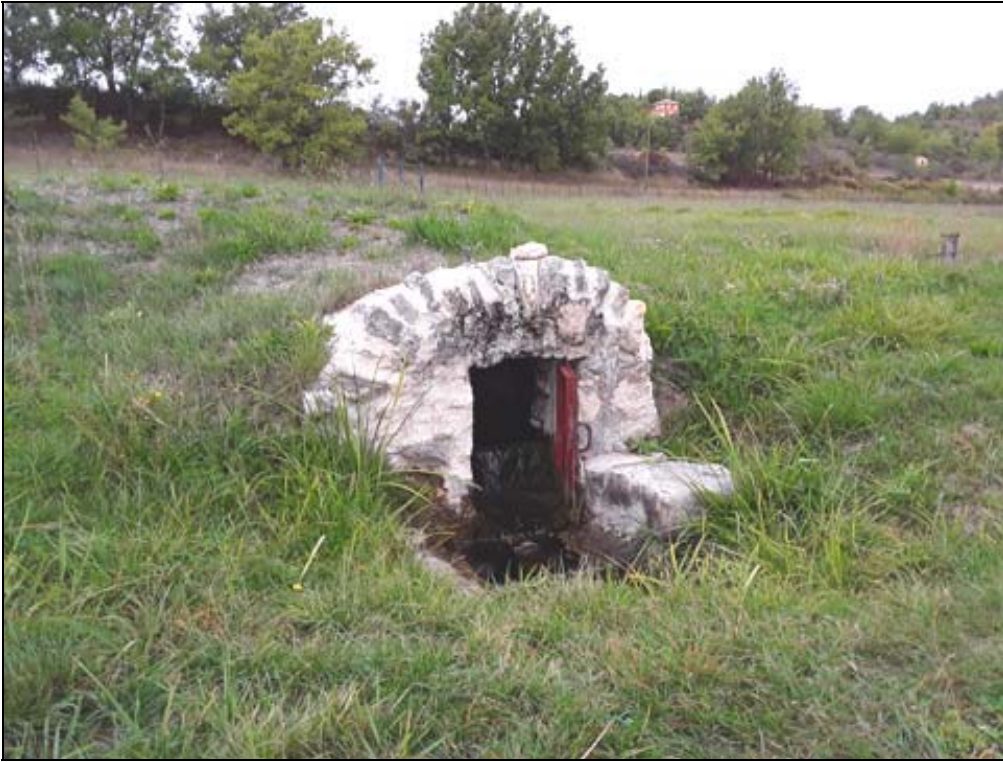
Station de surverse de la source.
